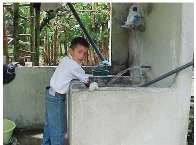
Water station, Colombia, photo credit: USAID.
